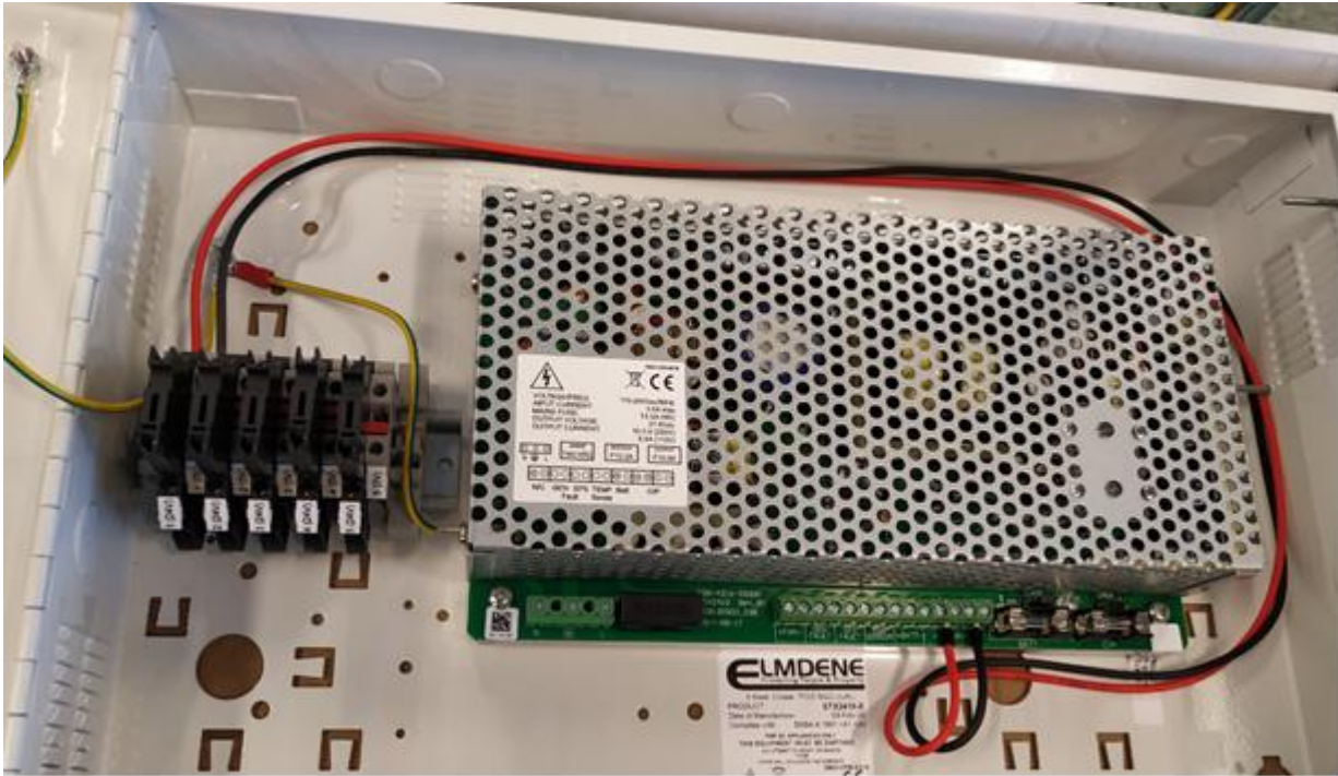
Figure 3: Example of setup for distributing 24 V power (the picture shows the 10A version).
